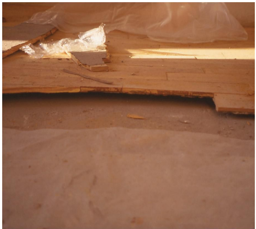
Buckling and tenting of the hardwood is common if the substrate moisture is too high. Photo courtesy of MAPEI.
