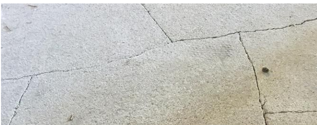
Vintage gypsum underlayment that presents wear, from mild to severe, is easily mitigated with a UL-certified gypsum repair protocol.
