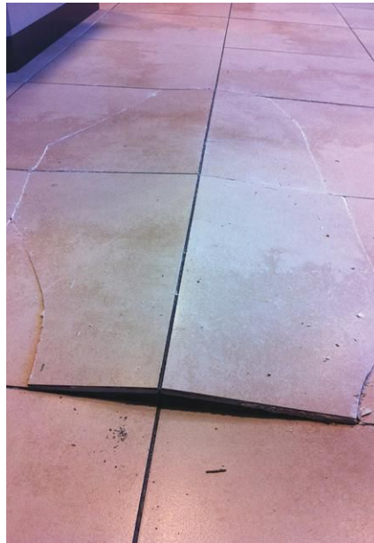
If the proper expansion joints aren't put in place, the tile will have nowhere to go during regular expansion and contraction cycles but up.
